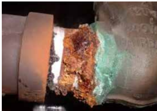
Figure 7: Pipeline corrosion damage
