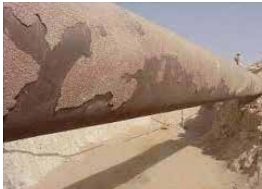
Figure 8: Pipeline corrosion damage
