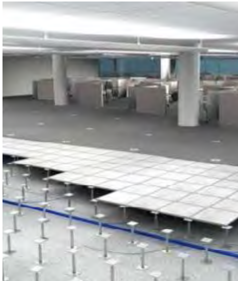
Largest Underfloor Air Distribution System (UFAD) - 2.5 Mn. ft2
